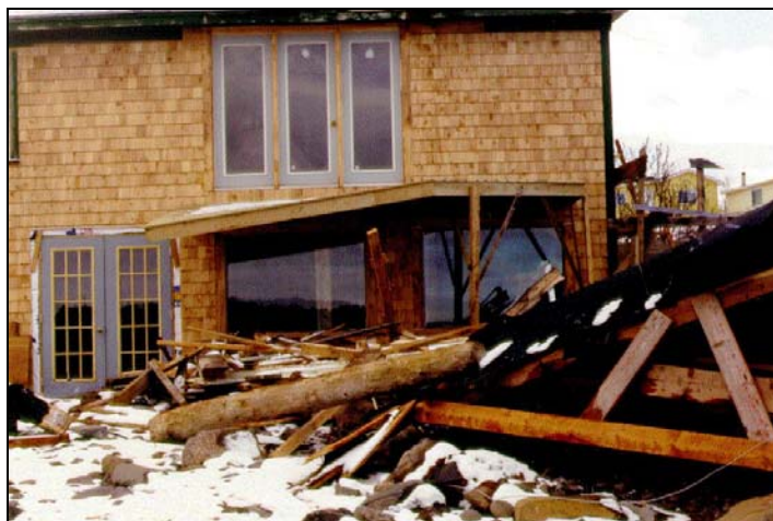
Figure 3. Photograph of storm-surge damage at Margaretsville along the Bay of Fundy coast in Nova Scotia.
